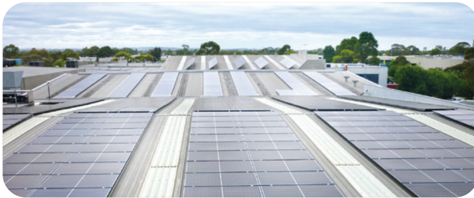
Solar panels implemented in Keysborough Site
