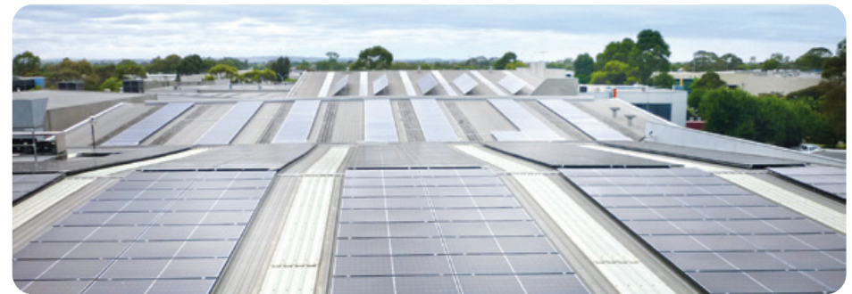
Solar panels implemented in Keysborough Site
